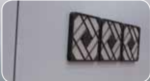
Inlet and exhaust fans with filters
